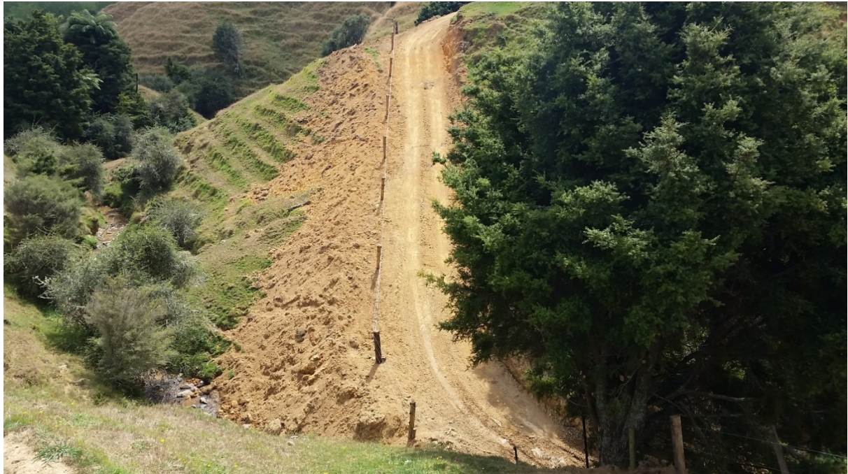
Figures 8 & 9: Bulldozed tracks for fence lines in hill country that are above streams
